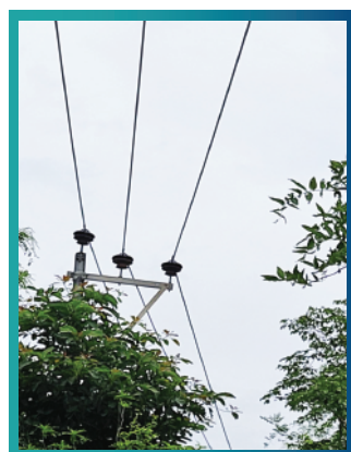
33 KV at KSEBL Kerla Evacuation Solar
