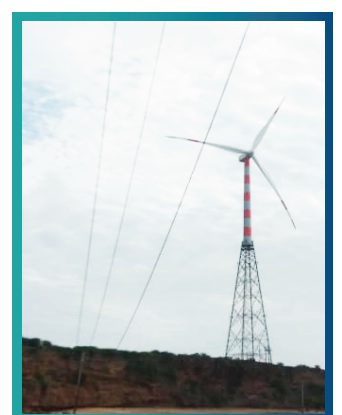
33 KV at TORRENT Bhavnagar Evacuation Wind Power
