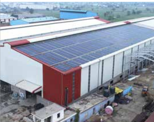
Salasar Techno Engineering, Pilkhuwa Capacity 560 kW
