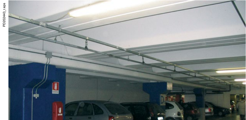
Canalis KBA supplying luminaires nearby sprinklers.
