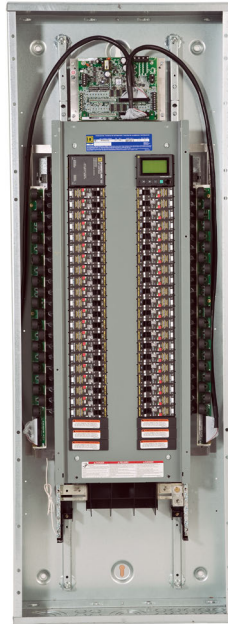
Powerlink Energy Management (EM) Lighting Control System
