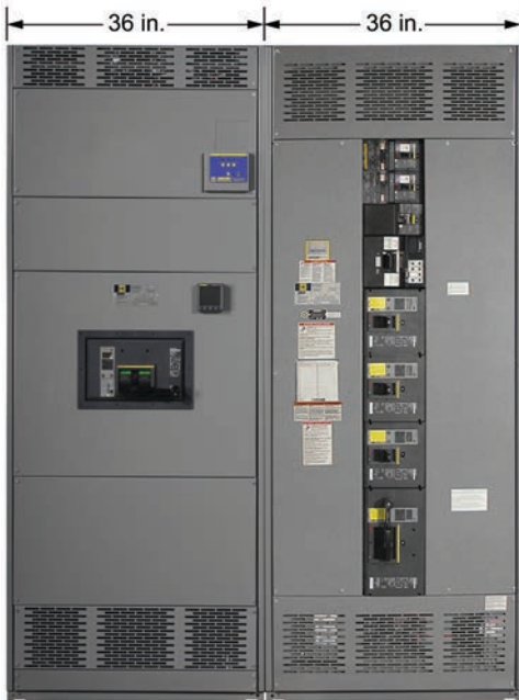
Shown is 2000 A, QED-2 Switchboard with 63 in. of Branch Circuit Breaker Mounting Height Available
