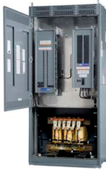
IPC2 Transformer Combo
