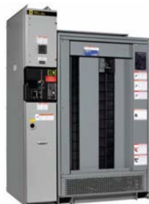
Model III Package Unit Substation
