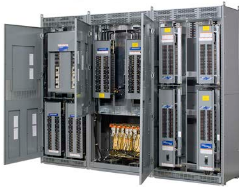
Integrated Power Center 2
